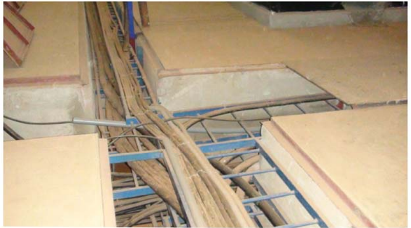
unattended cable trenches
