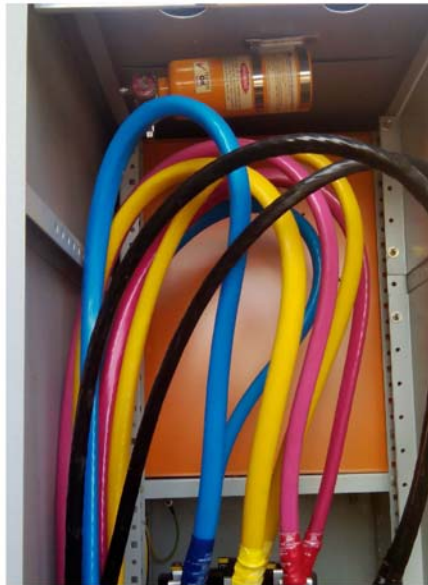
typical NASA 8T installation inside electrical panel
