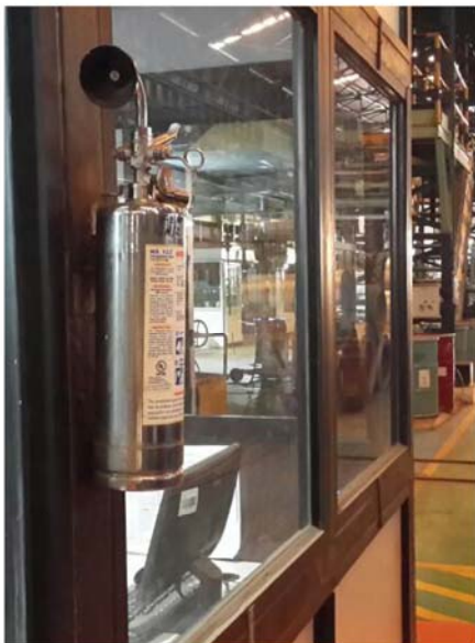
NASA 227 MAR installation at a steel coating unit
