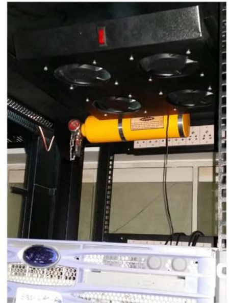
typical NASA 16T installation inside server rack
