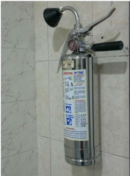
typical NASA 227 MAR installation in a hospital building
