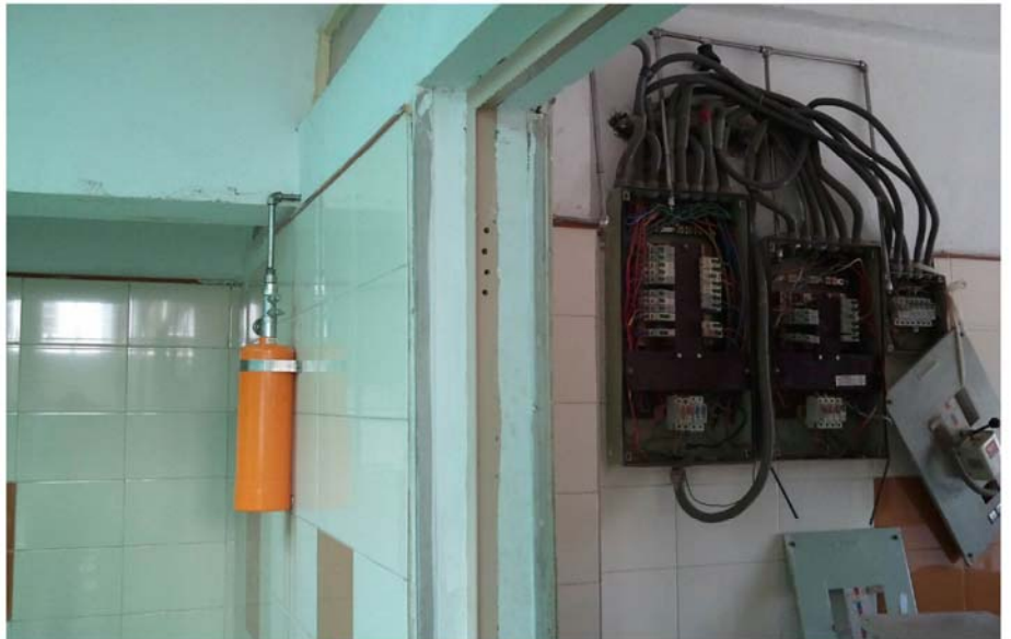
typical NASA fire suppression system for safety of electrical panels (in open condition)
