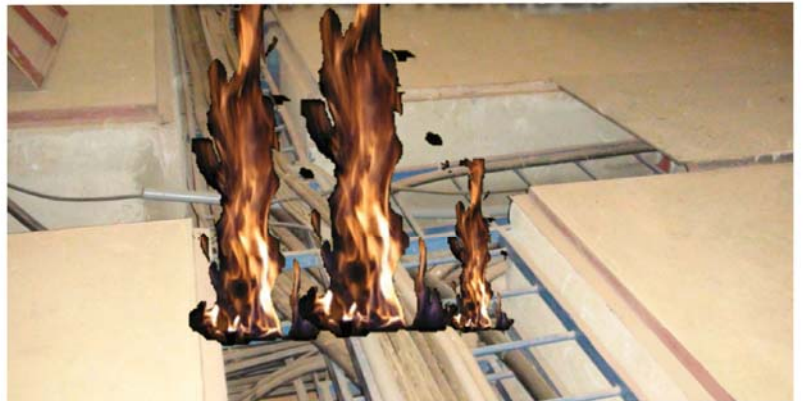
electrical fire leading to inferno
