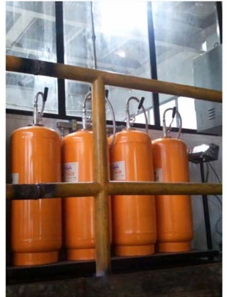
typical NASA fire suppression system for fire safety of a color coating unit
