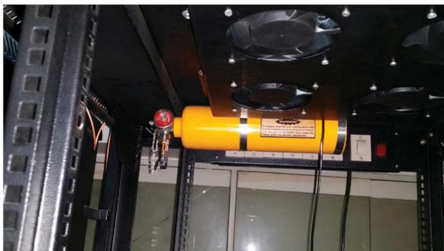
typical horizontal model installation inside server rack
