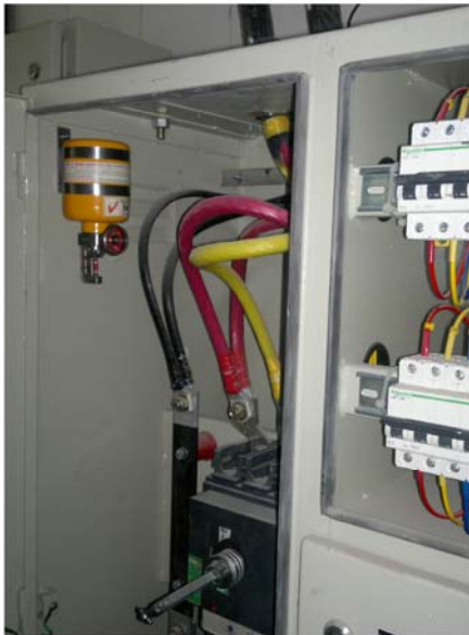
typical NASA 2T installation inside electrical panel
