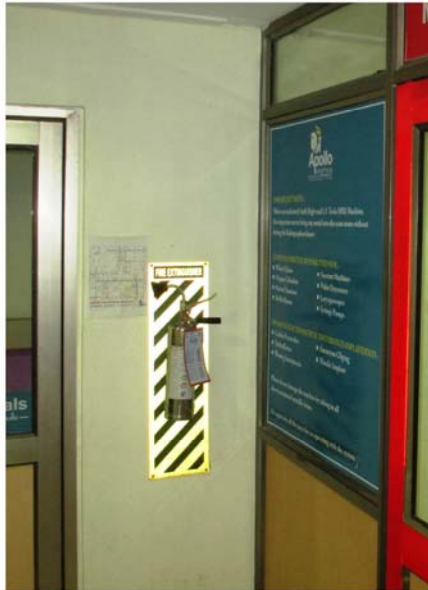
non magnetic NASA 227 MAR installed for fire safety of MRI machine at a hospital
